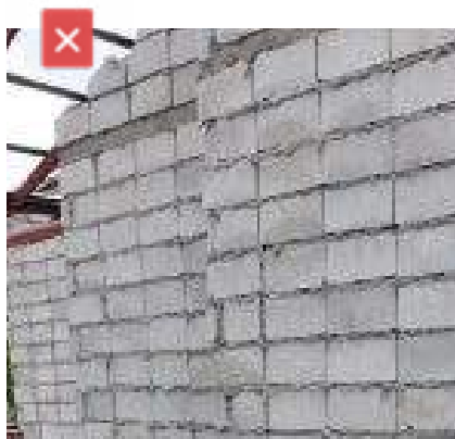
Placement not in a running bond
